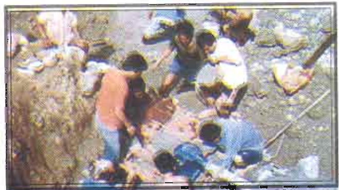
BSU-ANEC staff and some residents installing a 3-kilowatt microhydro system at Betwagan, Sagada, Mt. Province. An extension project of the College.
