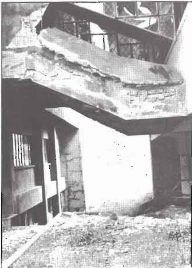
Stairs of the newly constructed Library Phase II sagged due to the earthquake
