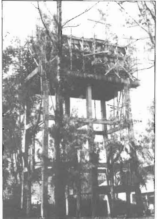
Foundation of the unfinished water tank and posts of the structure were damaged
