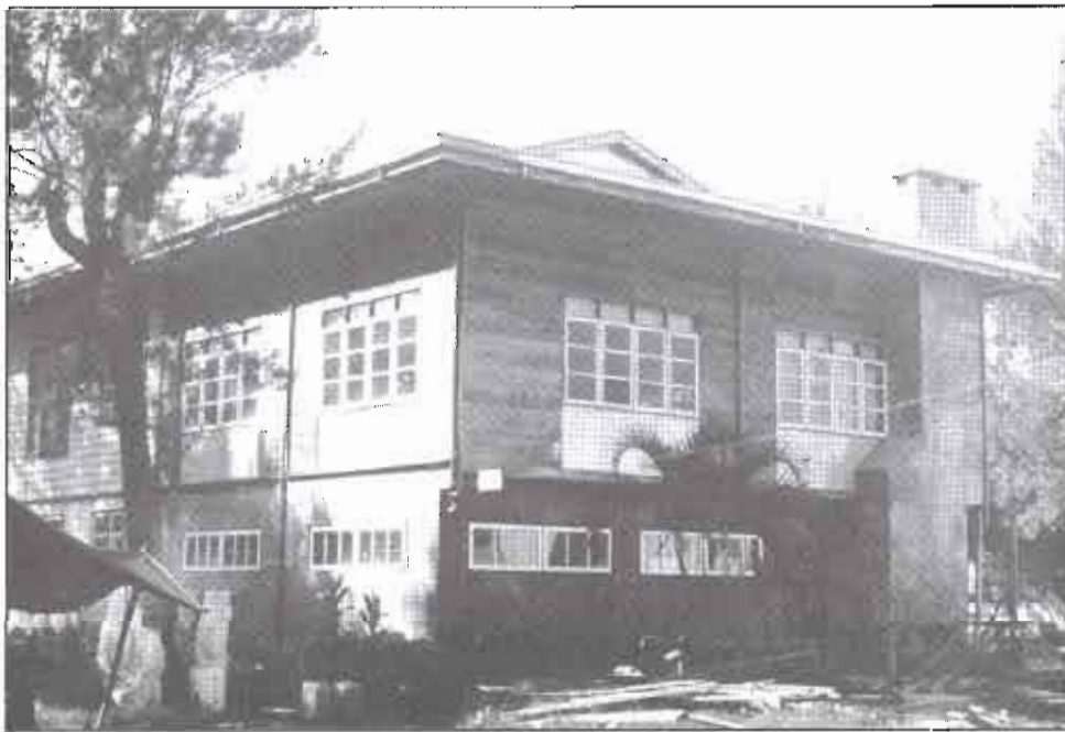
Extension & repair of the Home Economics Building. The hall on the second floor could be used for conferences, it could house 50 people.
