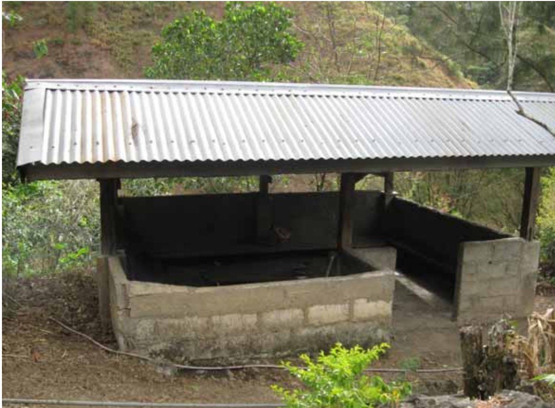
Figure 4. A modern abonan built out of blocks of cements, stones and green sheets
