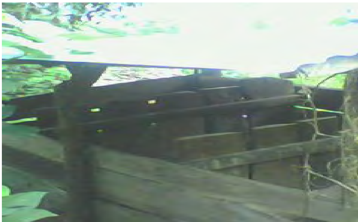
Figure 5. A pigpen having a G.I. sheet roof and wood walls owned by one of the respondent in barangay Macalana
