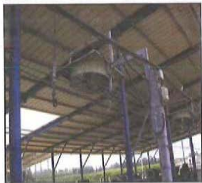
Figure 7. Center coolers ( Arnon farm)
